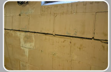
Horizontal cracking indicating bowing walls in basement
