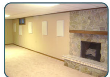
The SuperSump system utilized a bolted down air tight lid and high water alarm.
