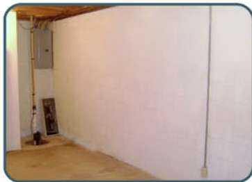
Bowing wall prior to installation. Existing sump pump in corner.
