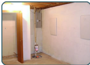
SuperSump installed and wall anchors with covers.
