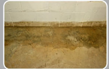
Water along the perimeter of the basement causing mold growth
